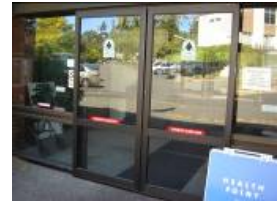
Automatic sliding doors are the preferred entrance
