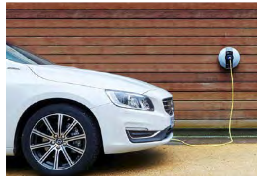
Figure 160: Parking for an electric vehicle.
