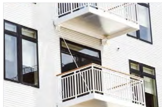
Figure 28: Examples of exterior supported balcony strategies that reduce thermal bridging potential. (3.3.1. b).
